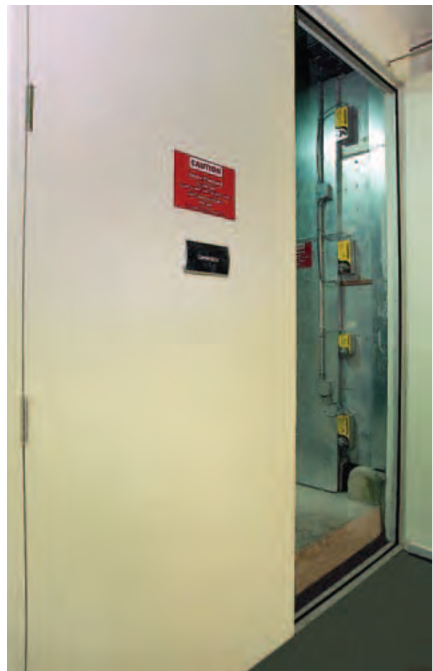
Metropolitan Hotel - Electromechanical Room
